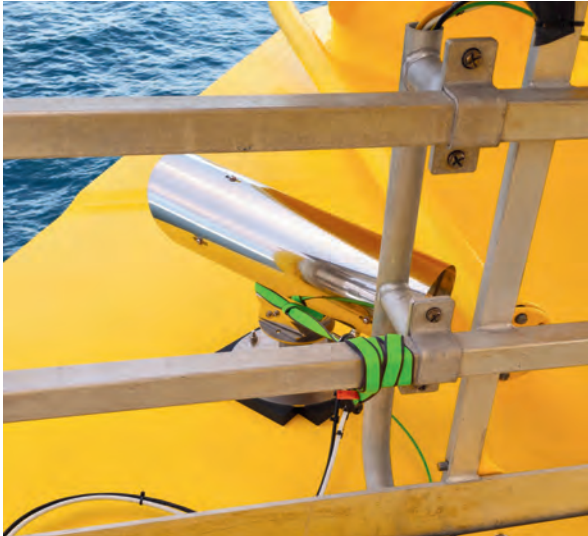
Spoor camera on Moray East transition piece
